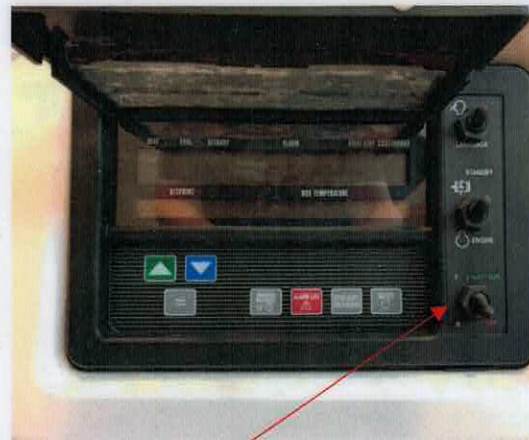
On/Off switch refrigerator
